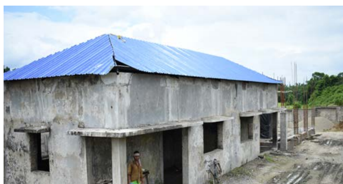
Water Treatment Plant in Hailakandi
