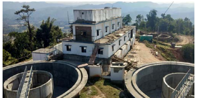
Water Treatment Plant in Dimoria, Kamrup
