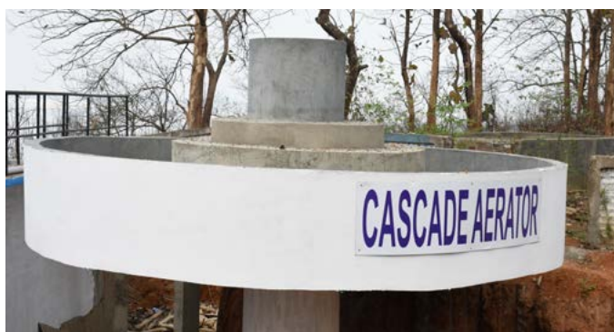
Water Treatment Plant in Chandrapur, Kamrup
