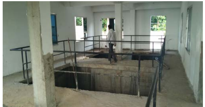
Water Treatment Plant in Dimoria, Kamrup
