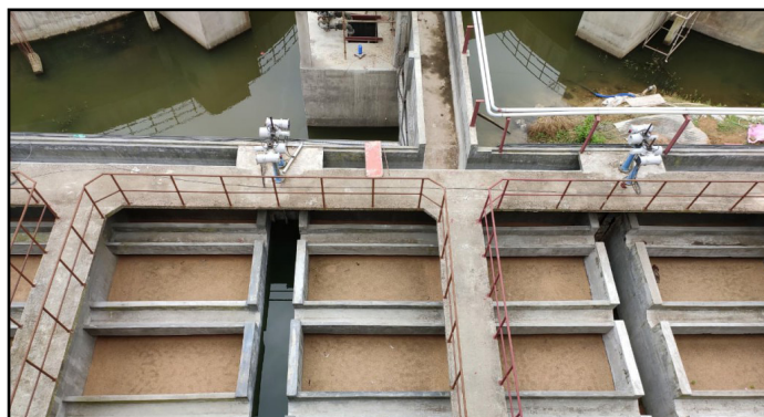
Water Treatment Plant in Jorhat
