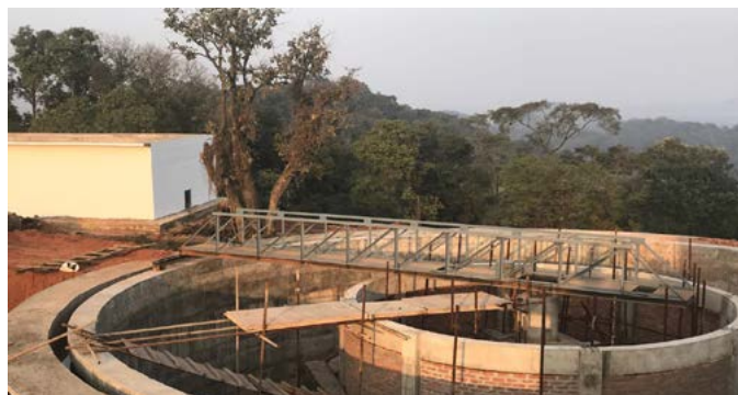
Water Treatment Plant in Dimoria, Kamrup
