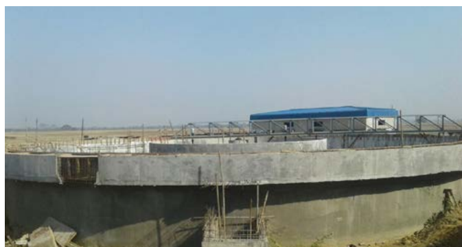
Water Treatment Plant in Jorhat
